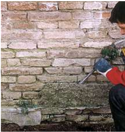
01 Remove the old render up to 1 meter above the damp line, exposing the bricks.
