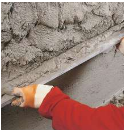
04 Apply the restoration render ADESAN CALCE INTONACO in a thickness of at least 2 cm.
