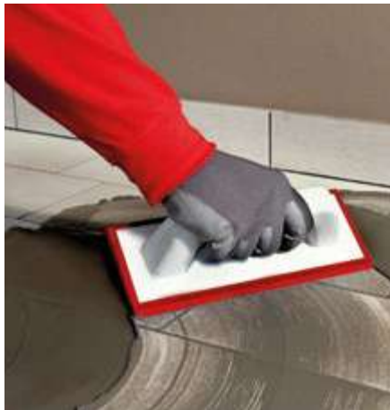
08 When the adhesive is dry, grout the ceramic tiles with the sealant ADEPOXY MATERIA , ADEPOXY MATERIA TECH , FUGAMAGICA 3-20 BIO MATERIA TECH or FUGAMAGICA ZEROSEI MATERIA .
