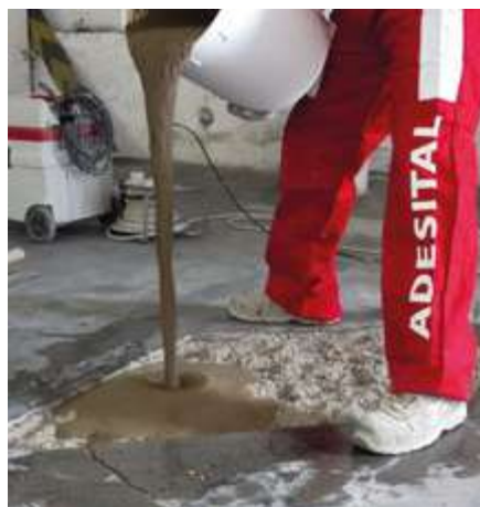
05 Application by pouring of ADEGROUT TRAFFIC in the area to be restored, taking care not to incorporate air into the mix.
