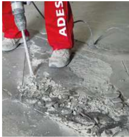
02 Mechanical removal of deteriorated concrete, oils, waxes and anything that may compromise product adhesion. Carry out these operations until you reach the substrate which is sound and with a rough surface.
