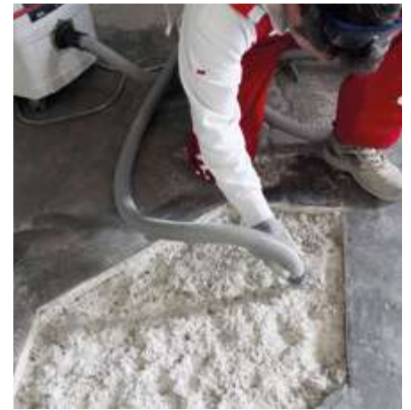
03 Careful removal of waste materials, vacuuming of dust and residues. It is important to work on a sound and perfectly prepared substrate, free of contaminants and materials from previous processes.
