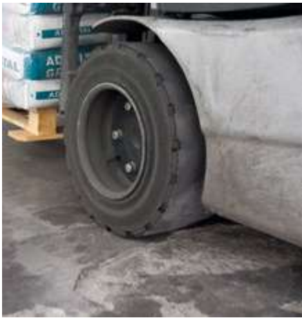
01 Damaged industrial floor that requires a rapid restoration with high strength.
